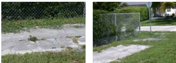
Figure 23. Broken and Missing Sidewalks
