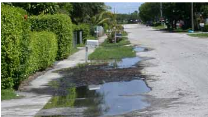
Figure 30. Localized Flooding in Swale Areas
