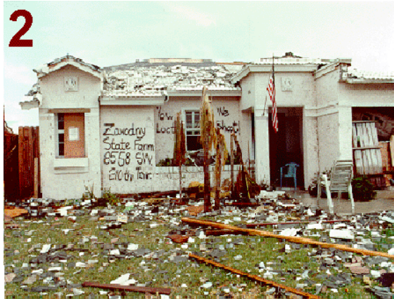
MAJOR DAMAGE HABITABLE
