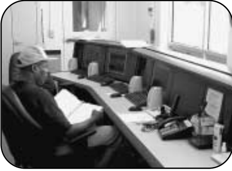
Monitoring the SCADA system at the Water Plant.
