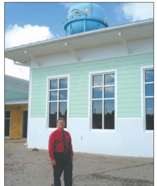
Environmental Services Director Richard Hasko is watching construction of the new building progress.
